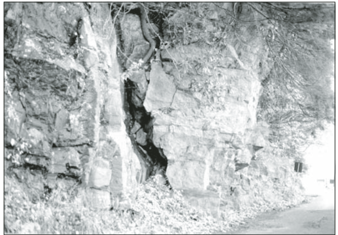
Figure 21. Irregular joints, trending along the Old Mine Road above the Karamac Trail. Boulders in the fractures are wedging the block apart, creating the potential for toppling.
