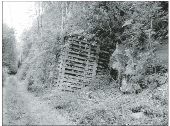
Figure 20. Concrete gabion along abandoned railroad grade below the Old Mine Road in Worthington State Park.
